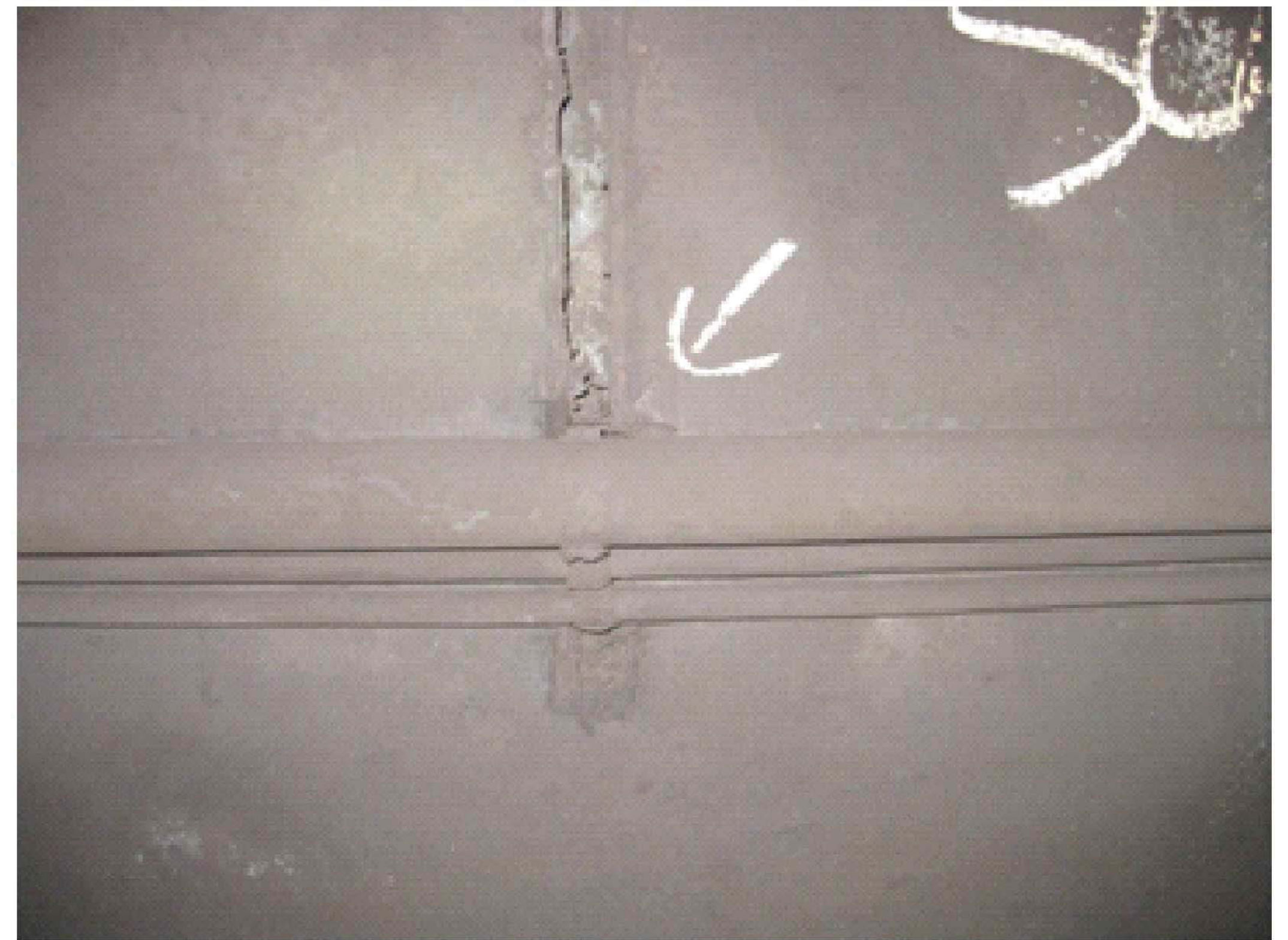
----- TYPICAL CABLES WITH BROKEN SUPPORT
