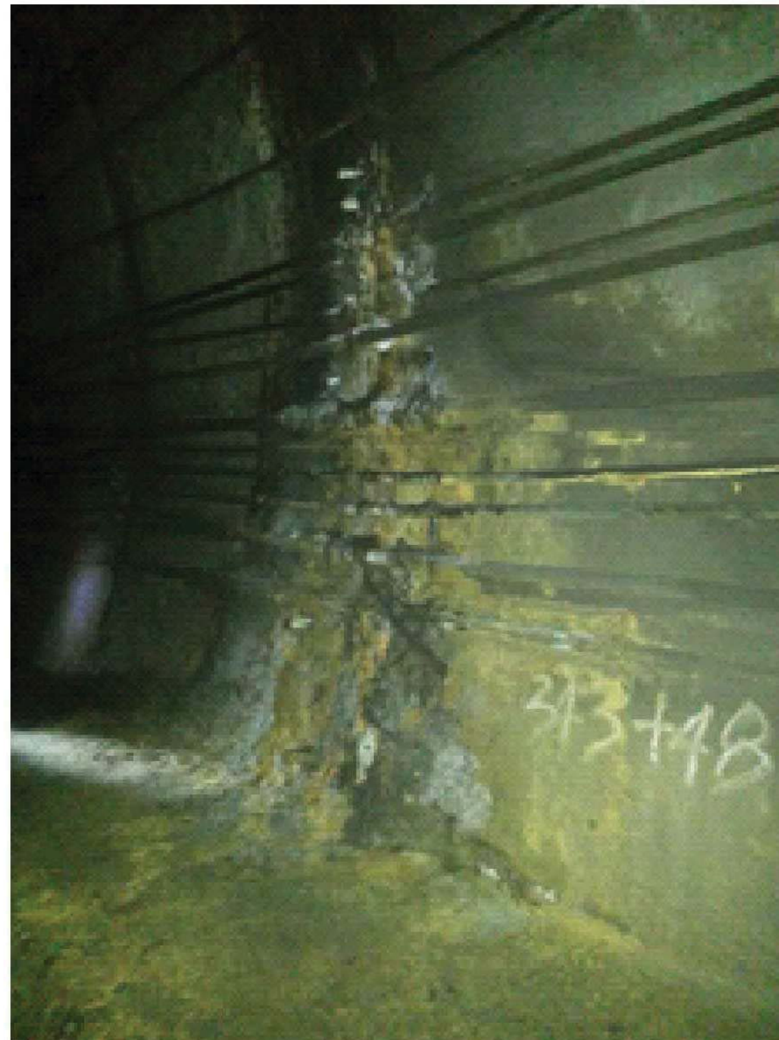
———— TYPICAL CABLES WITH VERY HEAVY CALCIFICATION
